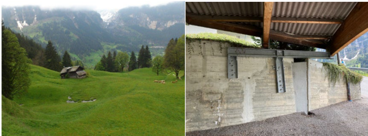
Figure 40. Photos from the Chratzera landslide report. Crack area of the landslide in Grindelwald (left) and repeatedly adapted garage roof in the village (right).
